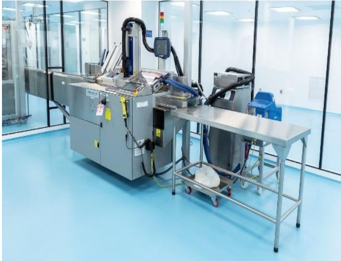
Tube filling equipment for semi-solid production line
