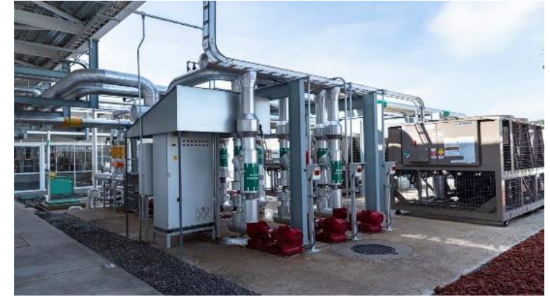
Water chiller system for OTC Plant
