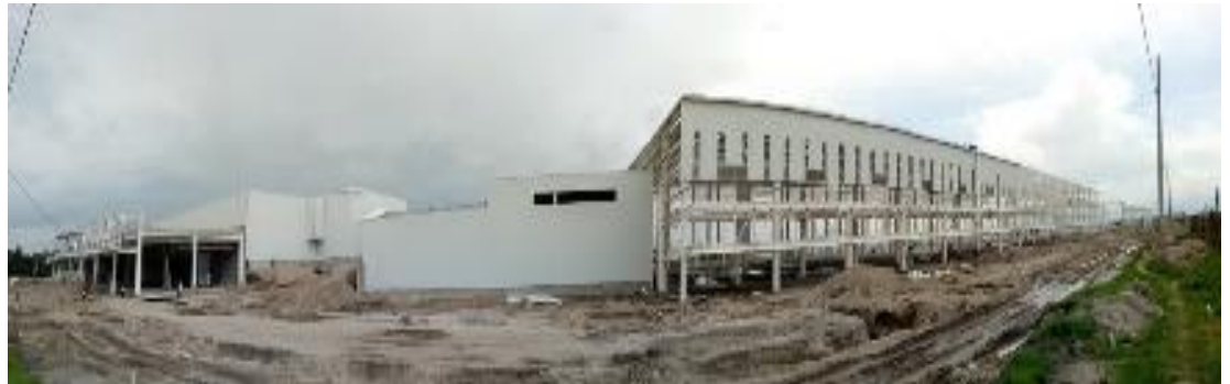
OTC Plant next to Finished Products Warehouse
